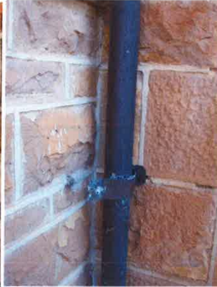
Photo 24: Loose downpipe bracket
