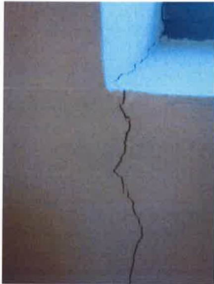
Photo 92: Room 4 cracking at window sill
