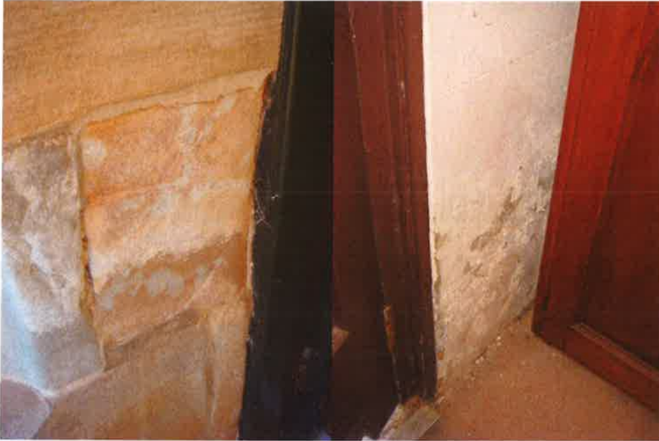
Photo 19: Salt attack and stone deterioration on the left side of the west porch doorway
