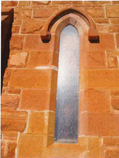
Photo 9: Typical lancet window showing cloudy protective polycarbonate cover
