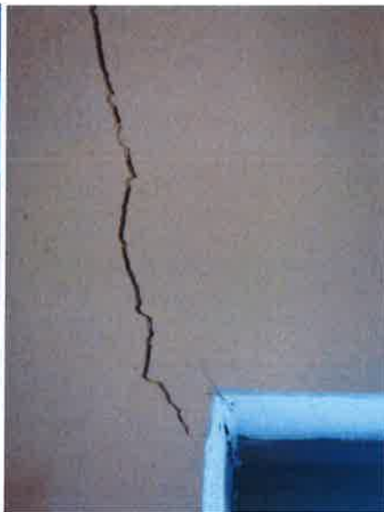
Photo 93: Room 4 cracking at window head
