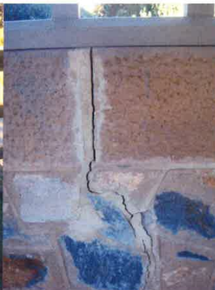
Photo 63: Evidence of past crack repair
