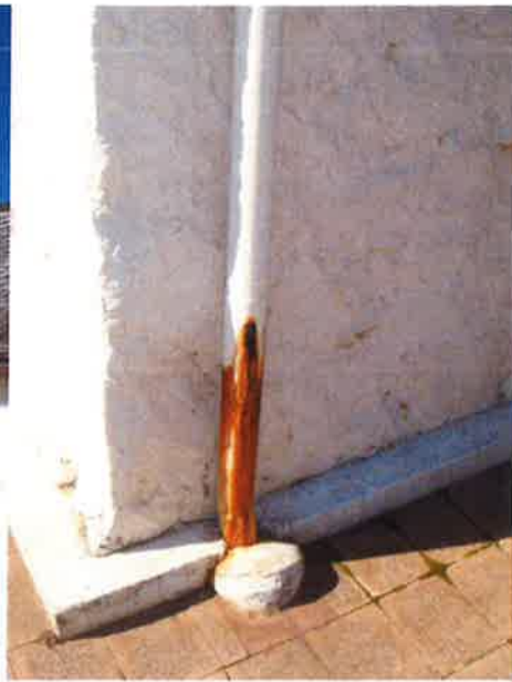
Photo 85: Leaking downpipe west side
