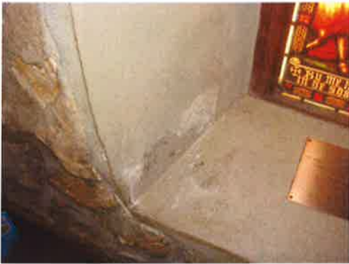
Photo 44: Moisture and salt attack at window sill in north porch
