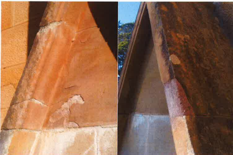
Photo 21: Typical stone deterioration at west side
