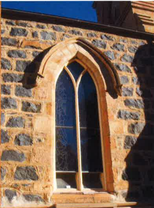
Photo 10: Typical window in original church nave. Note sandstone trims and label moulds
