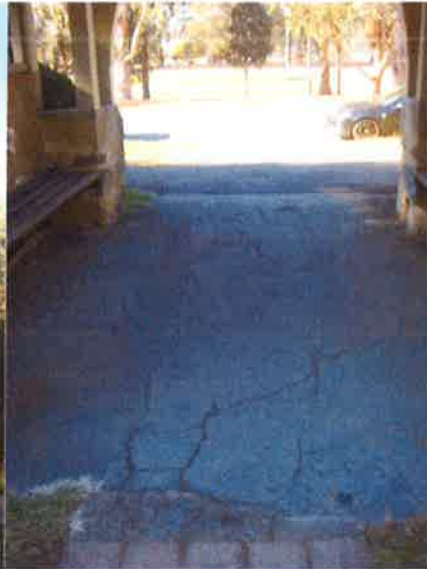
Photo 65: Cracked bitumen pavement
