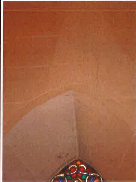
Photo 35: Typical movement cracks
