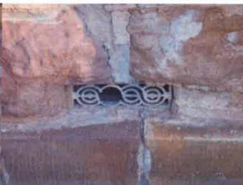
Photo 26: A broken cast iron sub-floor vent
