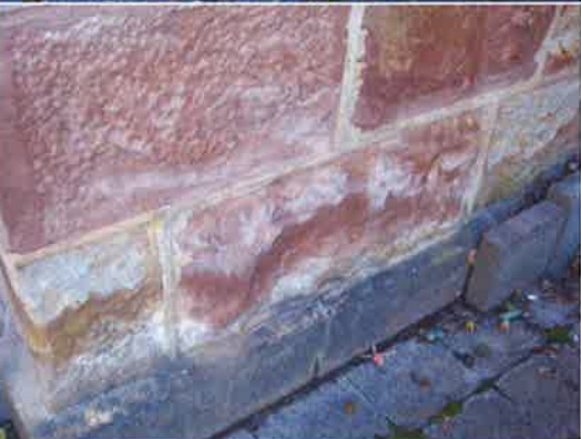
Photos 15-18 : Salt efflorescence at various locations around the building perimeter
