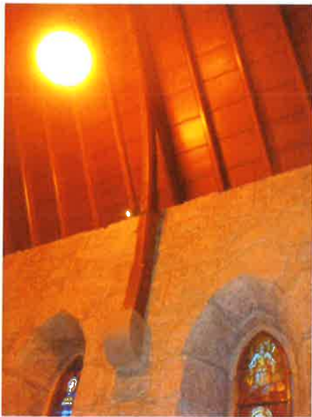
Photo 39: Chancel ceiling. The truss and corbel detail is simpler than that of the Nave
