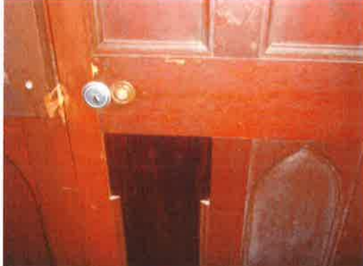
Photo 45: Damaged door under stairs in west porch
