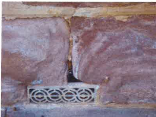
Photo 25: An example of highly eroded stone around a vent
