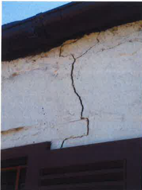
Photo 76: Moderate crack above south window
