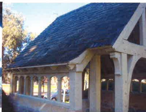
Photo 61: Roof detail showing weathered shingles
