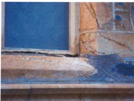
Photo 27: Failed apron flashing below window and poor re-pointing
