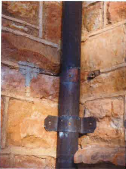
Photo 23: This downpipe bracket has been relocated inappropriately and the re-pointing has been poorly executed
