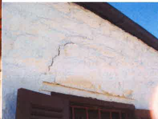
Photo 81: Minor crack above west side window
