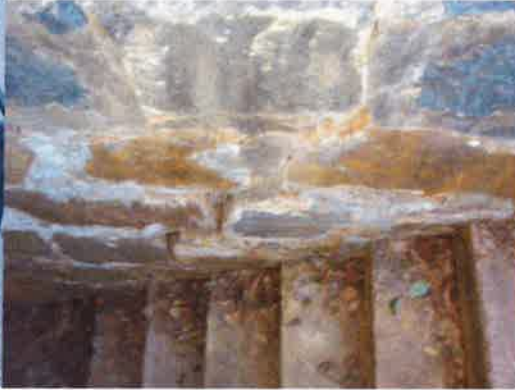
Photo 29: Movement in stone retaining wall
